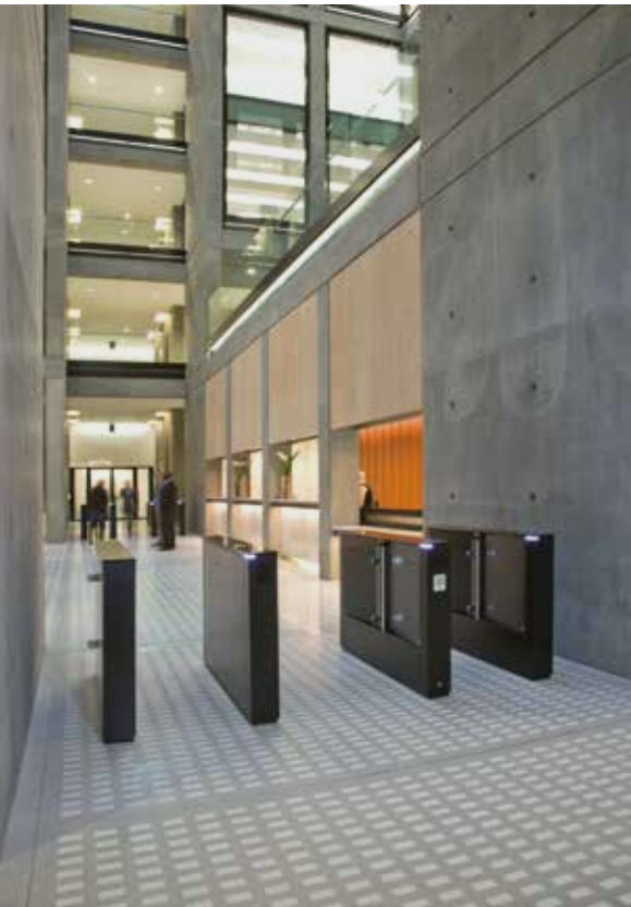
Access control turnstiles
